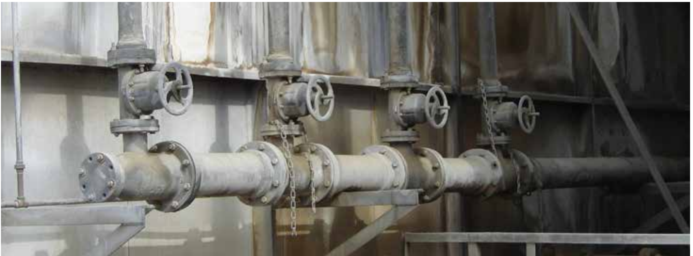
Straightway Rubber Lined Valves in Phosphoric Acid Service
